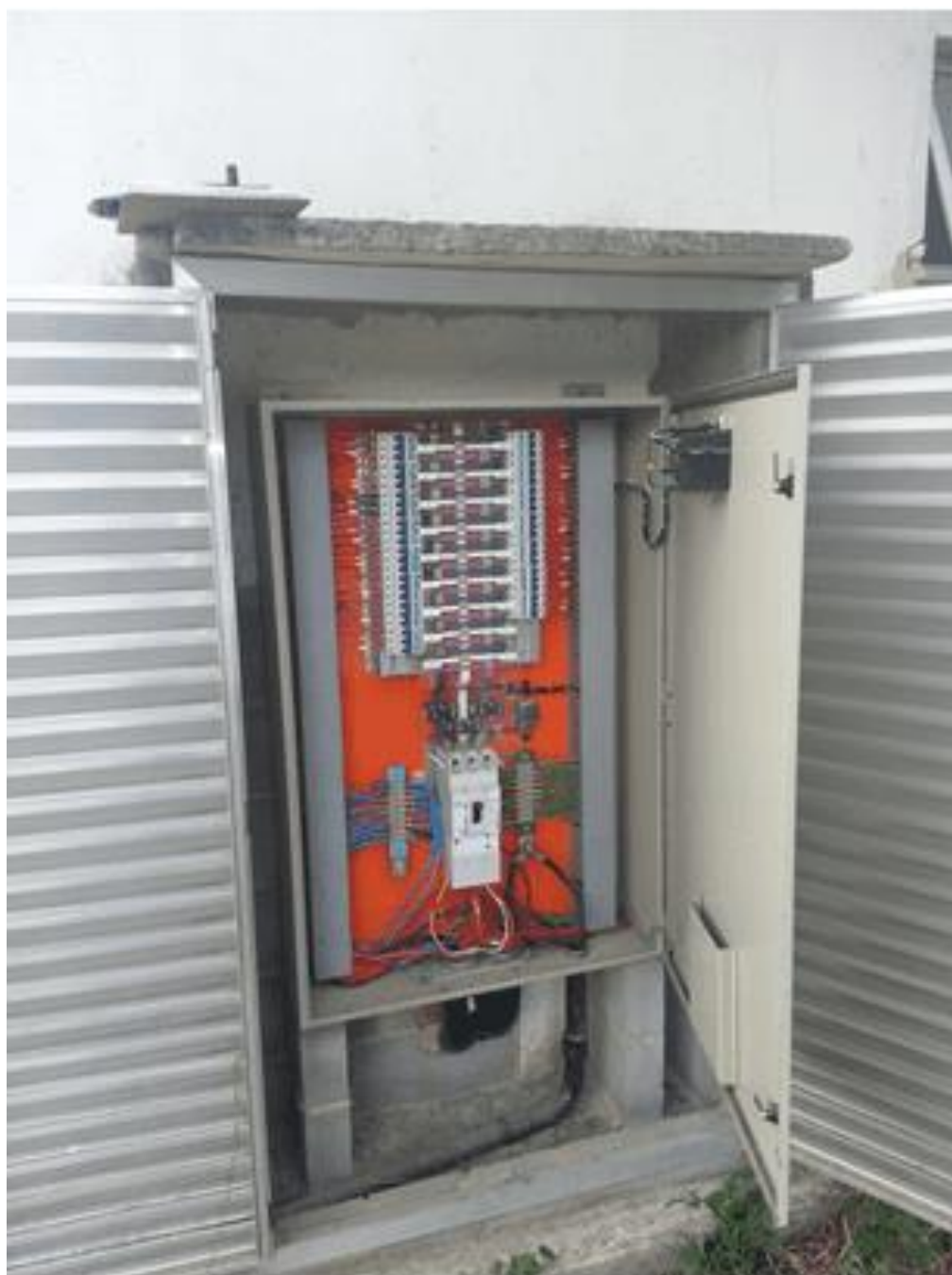
Figura 09 – Painel frontal do QGBT.
